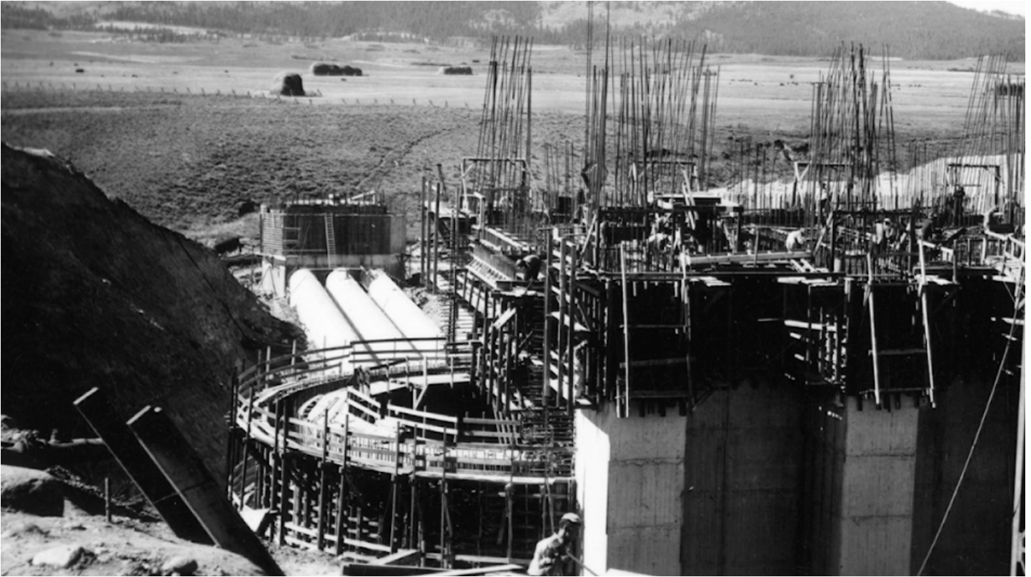
Crews construct the inlet structure to the Granby Pump Plant, which is now Farr Pump Plant.
