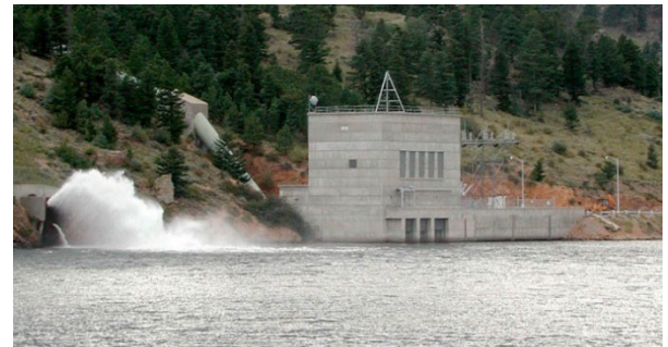
Mary's Lake Power Plant
