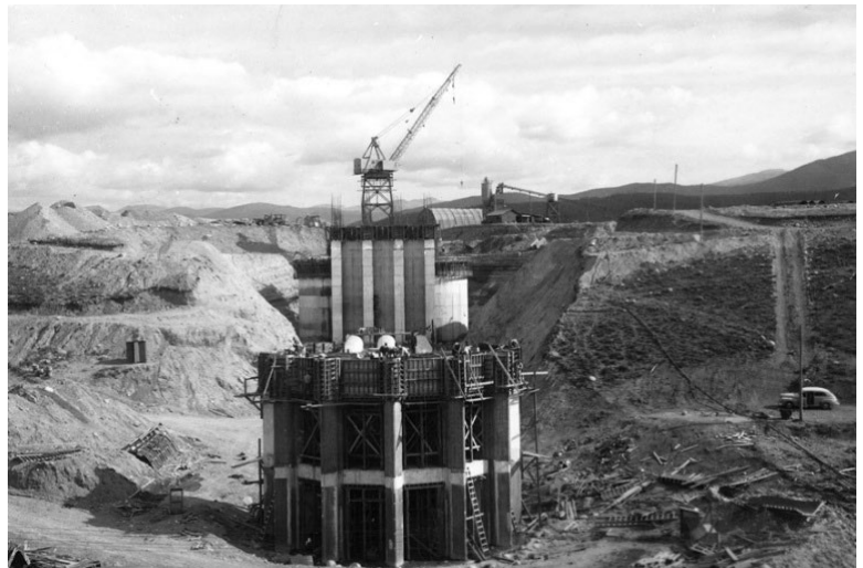
Building of the Granby Power Plant, which was later renamed the Farr Pump Plant.
