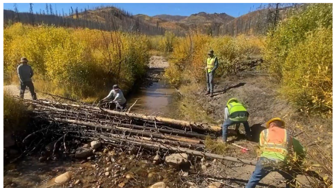
Crews placed post-assisted log structures (PALS) on Forest Service land within the burn area of the 2020 East Troublesome Fire.
