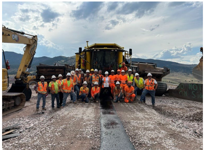
The final lift of asphalt was placed on the main dam on July 18, 2025.
