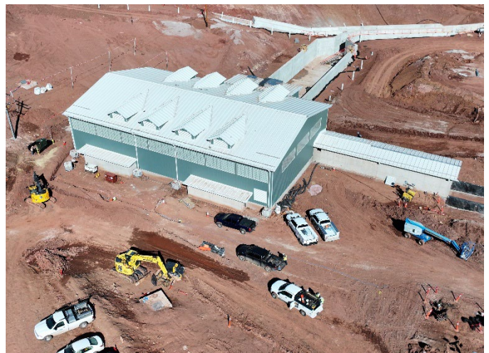
The valve house will control pressures and flows between the C-BT Project and Chimney Hollow systems.
